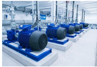
Maintenance, supervision (station de pompage, autoroutes ...)
